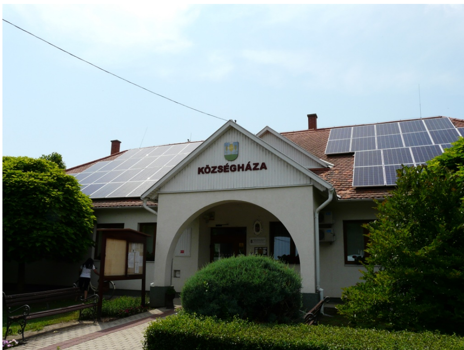
PV panels on the building of the Town Hall in Nagyhegyes
